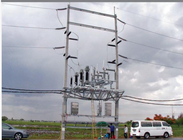
Figure 1. Switching station using Series 2000 Circuit-Switcher.
