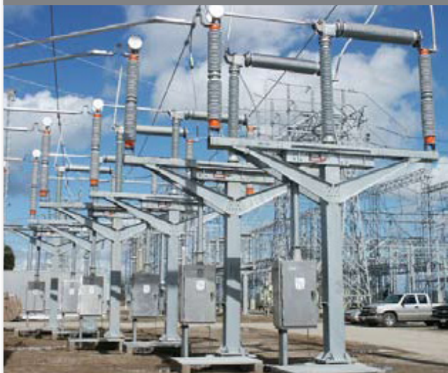
A Series 2000 Circuit-Switcher protecting a single-phase reactor.
