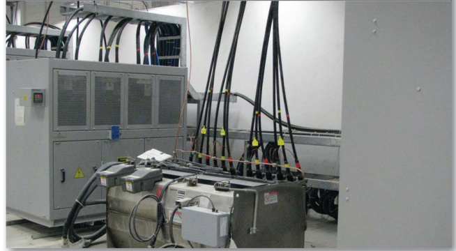
Installation of a Remote Supervisory Vista Underground Distribution Switchgear unit.
