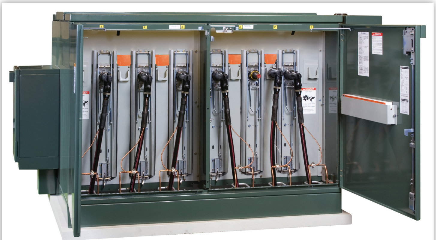
FIGURE 4. Remote supervisory PME Pad-Mounted Switchgear with fuse compartment open
