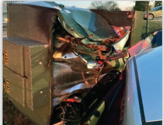
FIGURE 3. The aftermath of a vehicle colliding with one of Ameren Missouri's pad-mounted switchgear units.
