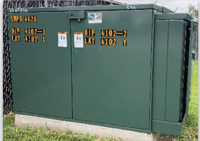
FIGURE 1. An S&C Remote Supervisory PME Pad-Mounted Switchgear unit that is boosting Ameren Missouri's reliability and resilience.
