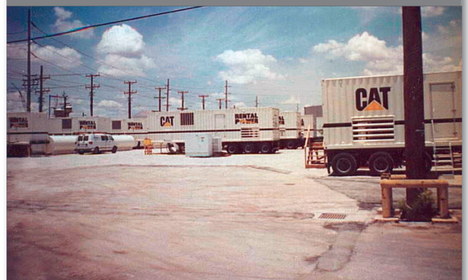
A 30-unit generator farm.
