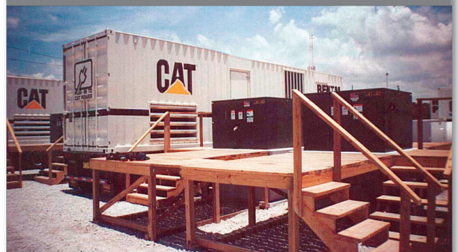
Two pad-mounted gear units are located between two generators (generator on right is not visible).
