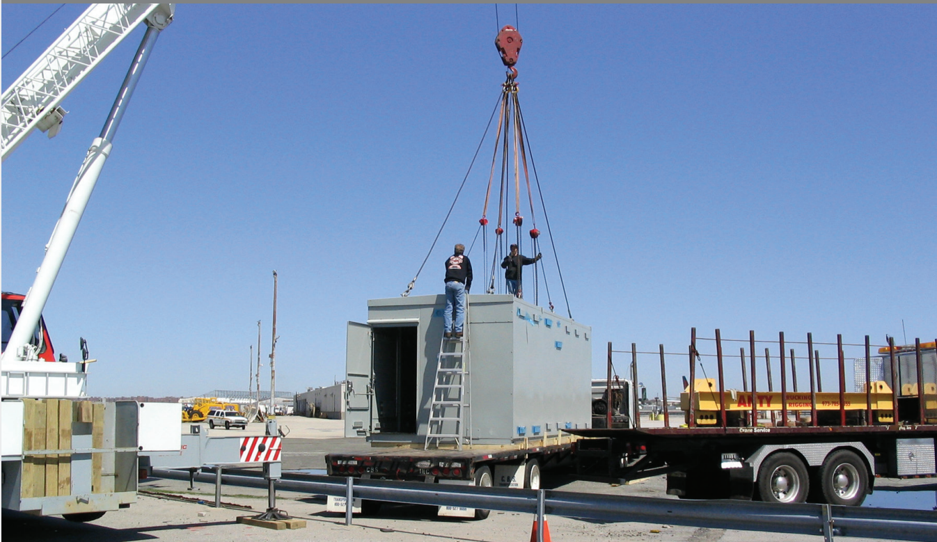
Pre-assembled gear was lifted and placed in one piece in under one hour.
