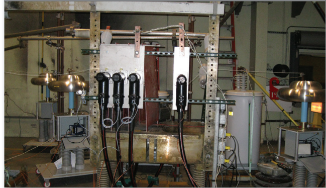
Figure 3. Test stand with one faulted phase elbow and three unfaulted phase elbows with faulted-circuit indicators mounted.
