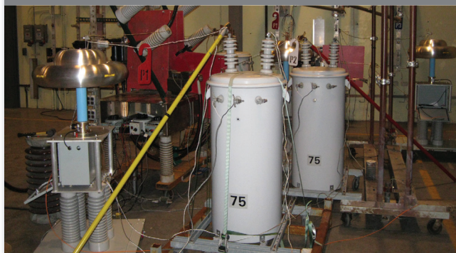
Figure 1. Circuit setup showing use of distribution transformers to energize unfaulted phases having faulted-circuit indicators.
