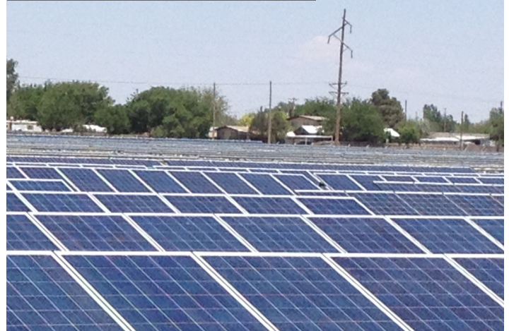
2.5-MWs of PV Solar Panels at the Roswell Solar Plant
