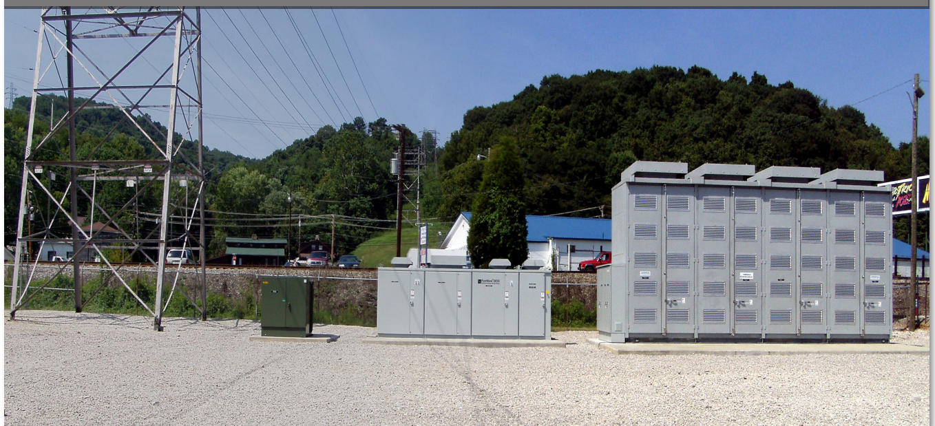
Distributed Energy Storage System.
