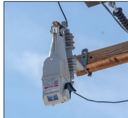
TripSaver® II Cutout-Mounted Recloser (Also West Palm Beach)
