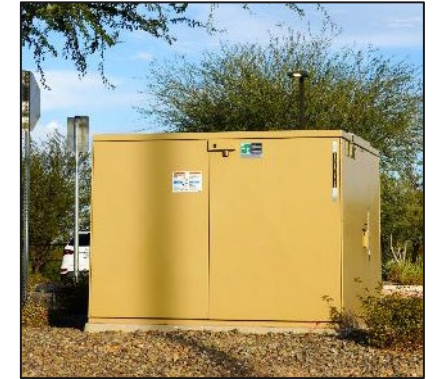
PME Pad-Mounted Gear
