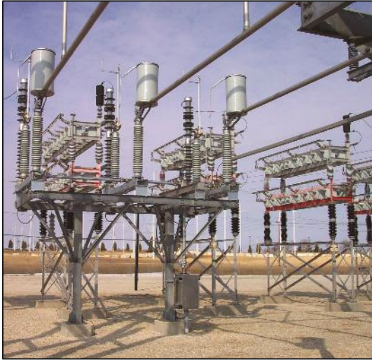
Mark VI Circuit Switcher
