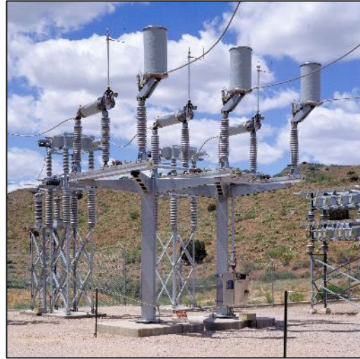
Mark V Circuit Switcher
