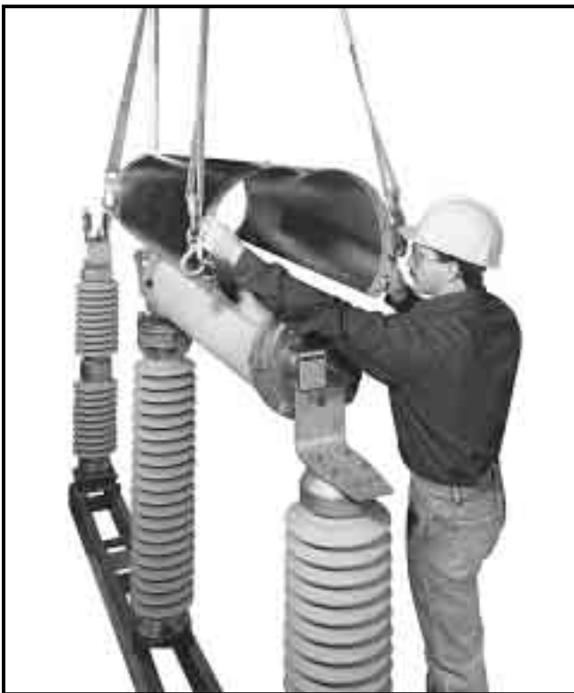
Figure 9. Raising spare interrupter container into position on interrupter being replaced. Model 2010 Circuit-Switcher illustrated; Models 2015 and 2040 are similar.
