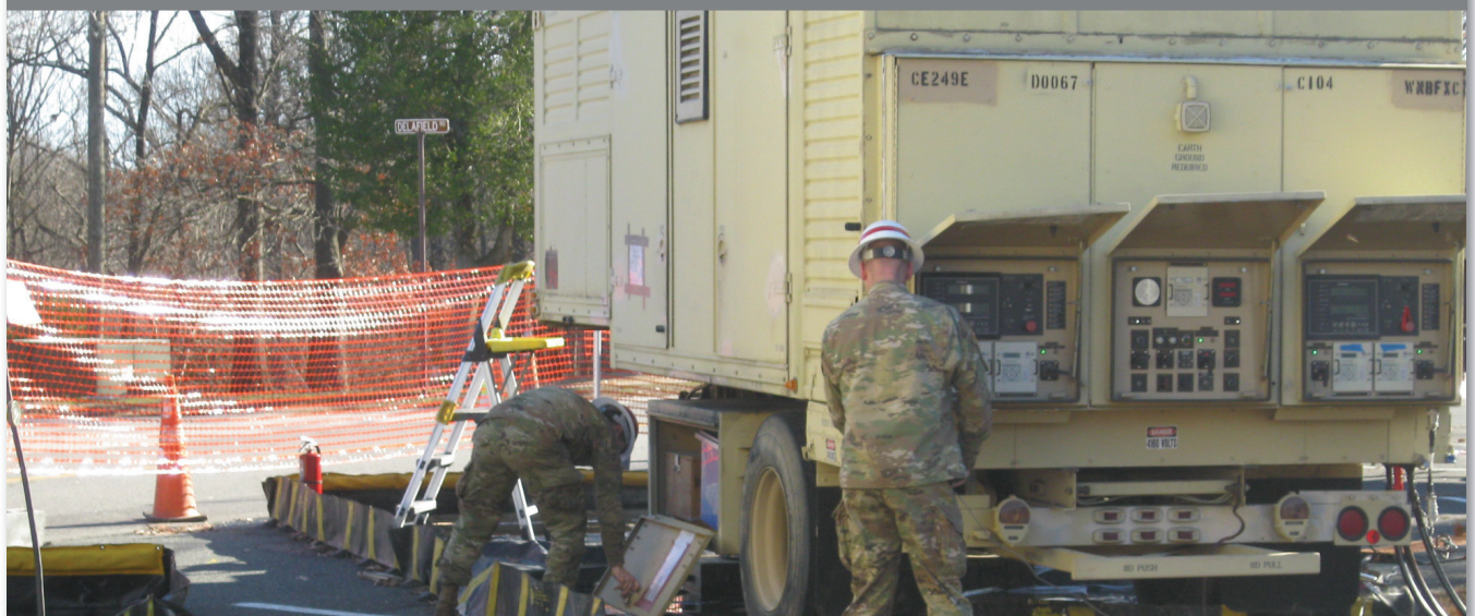
Testing and commissioning of a mobile generator integrated into the microgrid at Fort Belvoir.
