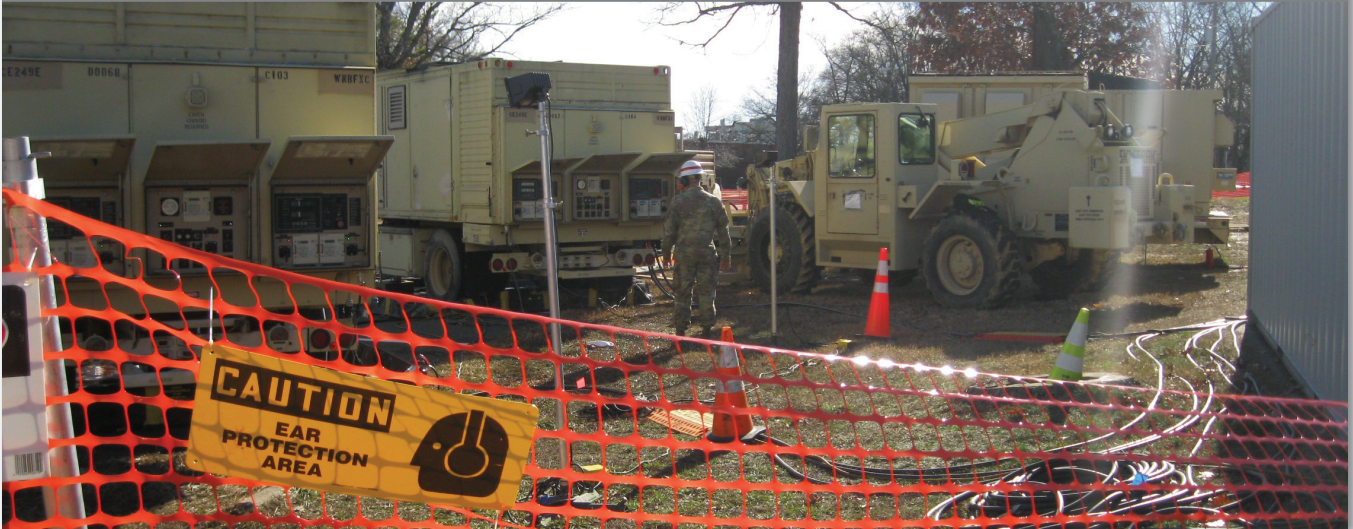
Monitoring the mobile generators during microgrid operations.
