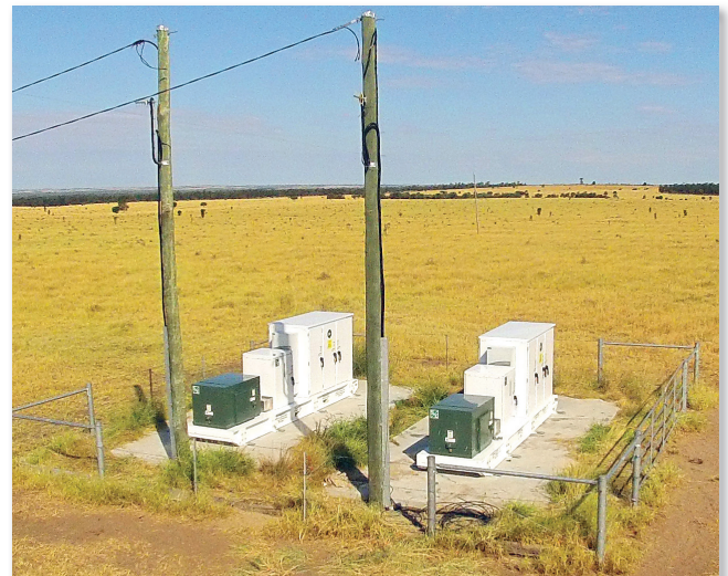
Twin Grid Utility Support System units providing extra support along a SWER line.
