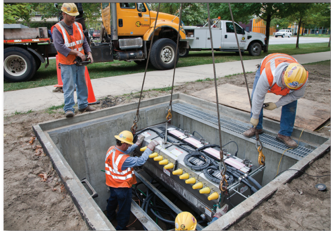
Installation of S&C UnderCover™ Style Vista Underground Distribution Switchgear.
