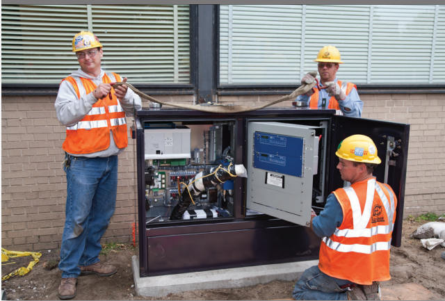
Installation of S&C Remote Supervisory Vista Underground Distribution Switchgear for a High-Speed Fault-Clearing System.
